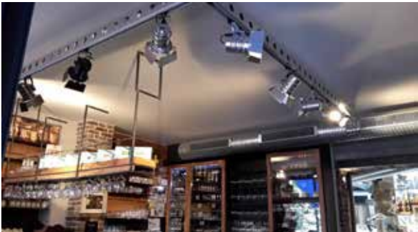
Trattoria Restaurant U-Match; Duct France
